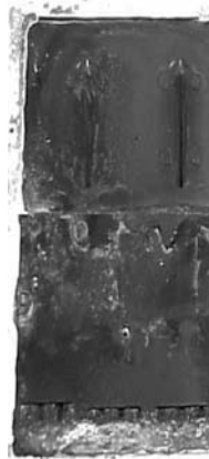
Example 1: Corrosion on cold spot baffle
